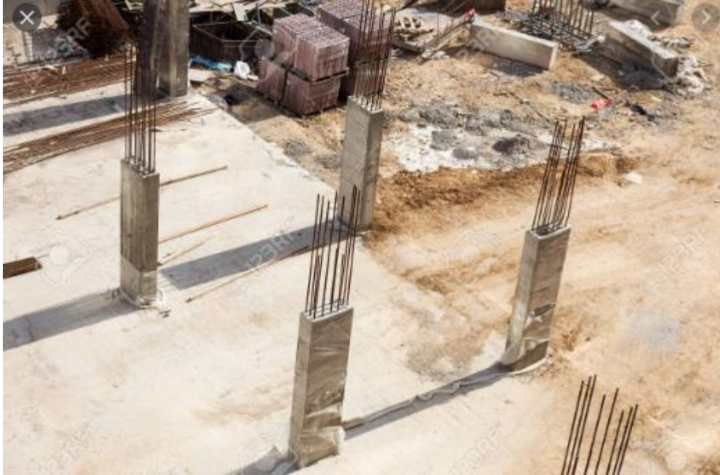
Figure 167: Concrete by letting it dry and carry out curing Source: Design building.com – foundation construction building site.
