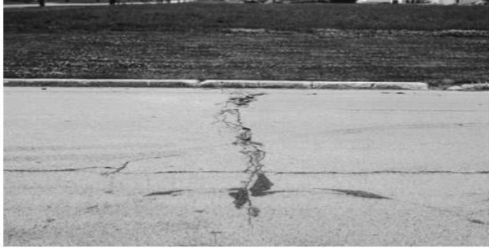
Figure 143: longitudinal and transverse cracking
