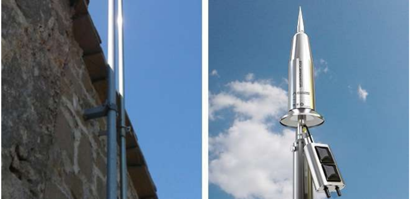
Figure 53: Lightning rod image
