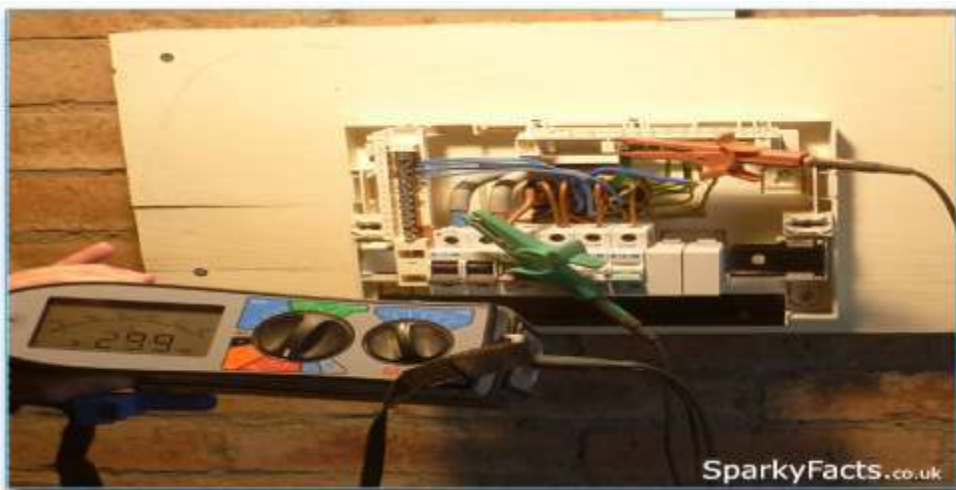
Figure 322 Insulation Resistance test sequence
