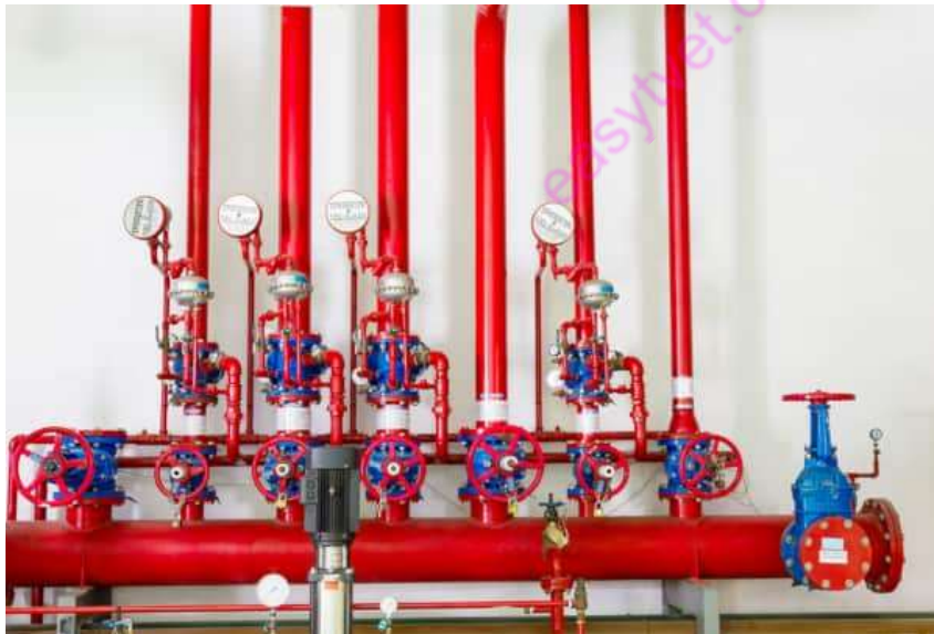
Figure 186 - Fire Control Piping Appliances
