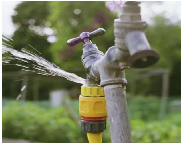
leaking hose bibb
