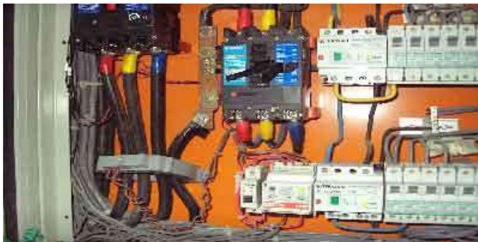
Figure 9: industrial main switch
